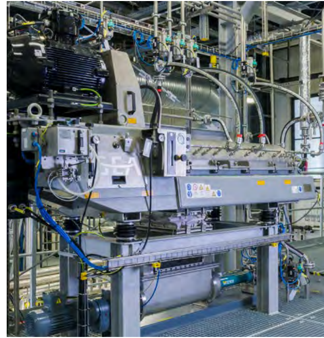
Decanter for the separation of fine and suspended particles
