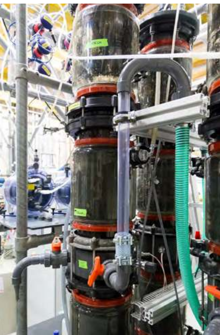
top: One-stage high-load digestion plant in Ilsfeld
